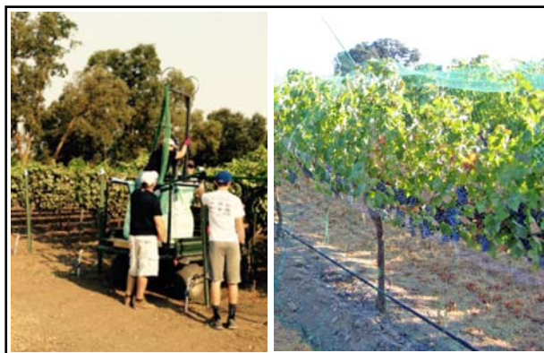
Lynne Poole had her father fabricate their own Applicator Platform to fit in the back of a utility vehicle. It cut installation time dramatically.
