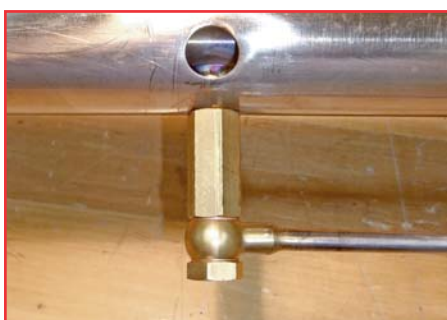
Start the fogger to check for leaks. If it does leak, carefully tighten with wrenches.
