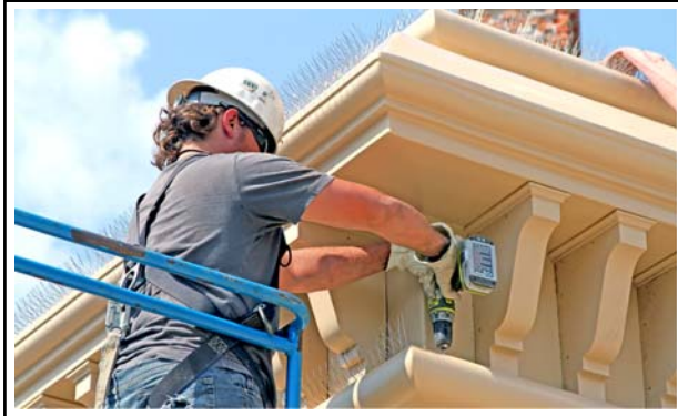
Once the new tower section was on-site, the installer cleaned & prepped all the installation surfaces and began installing the Premium Nixalite Spikes.
