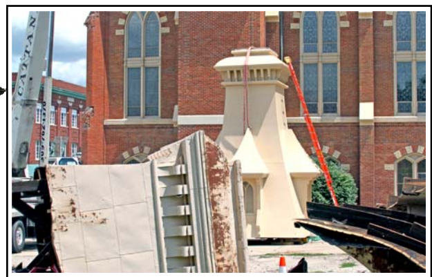
The old tower (foreground) had to go. The new tower (made by Fiberglass Specialties, Henderson Texas) was ready but still needed bird spikes.
