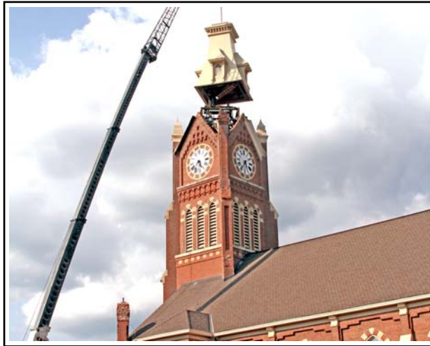
The First Lutheran Church was replacing the top section of their bell and clock tower. Before the new one went back up, they had to do something about the pigeons that had contributed to the original problem.
