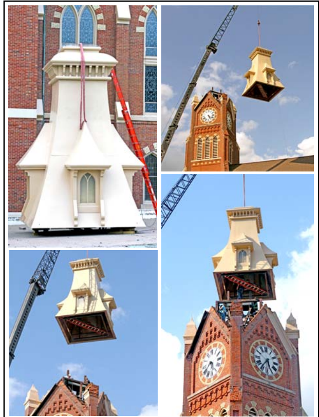
After all the Premium Nixalite spikes were installed, the new tower section was rigged and then lifted into place atop the main clock & bell tower.
