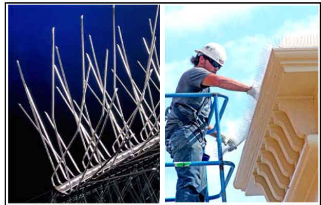
After considering all of the installation requirements, both Nixalite and the First Lutheran Church agreed that the best choice for permanent bird control would be the All Stainless Steel Premium Nixalite Bird Spikes.
