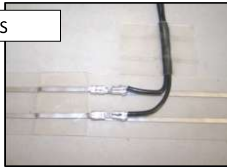
A single pair Splice Tap with wires secured by scrap tape.
