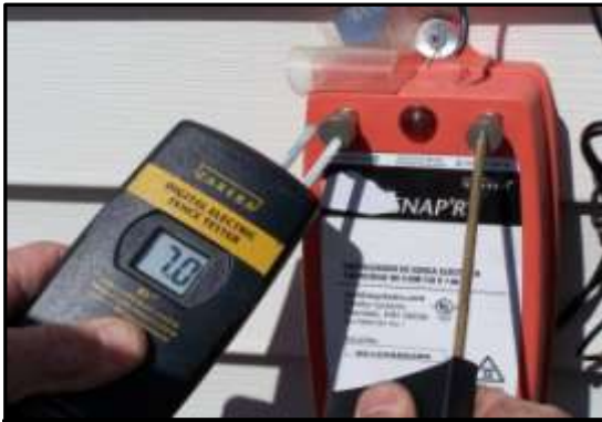
Reading voltage of the line charger while disconnected from the system.
