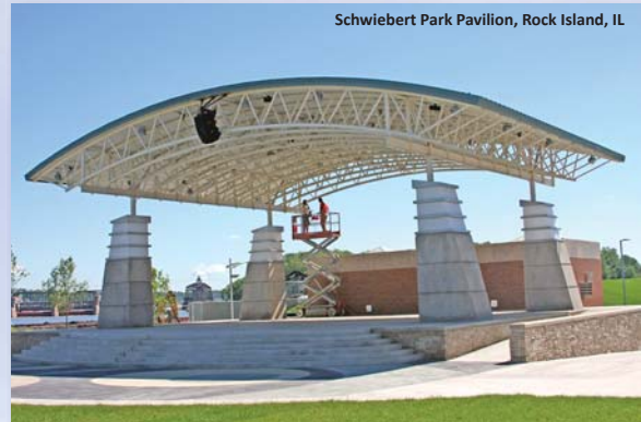
This pavilion's open steel framing offered birds safe harbor. After careful observation and measurement, K-Net was installed with a cable system to keep birds out and surfaces clean.
