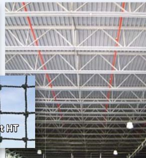
The black K-Net blends in with the gray roof decking behind
